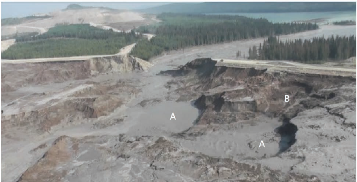
FIGURE 5.1.2: VIEW LOOKING DOWNSTREAM SHOWING UPSTREAM SIDE OF DAM AND REMAINING TAILINGS
