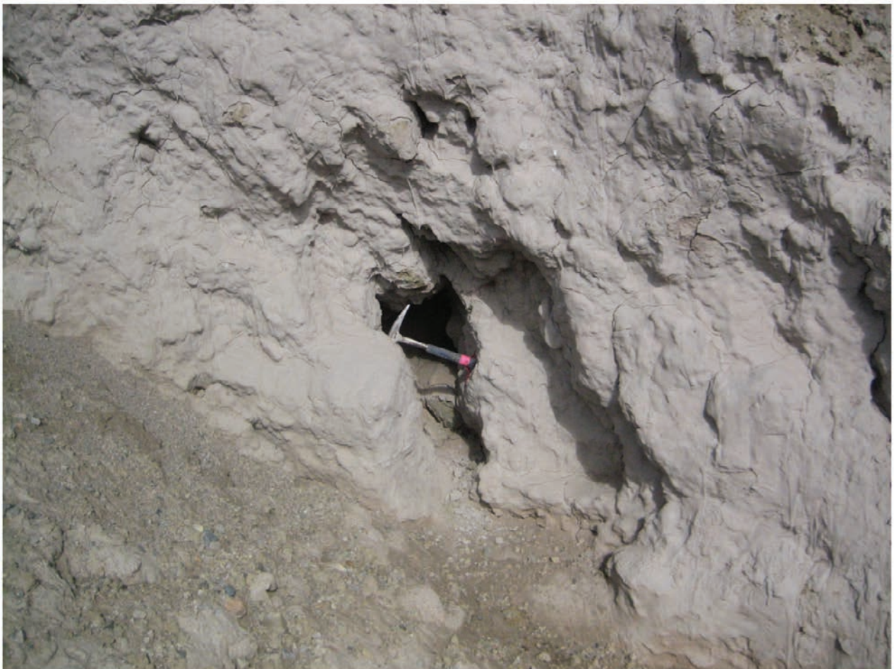
FIGURE 5.1.8: VOID ON UPSTREAM SIDE OF LEFT ABUTMENT
